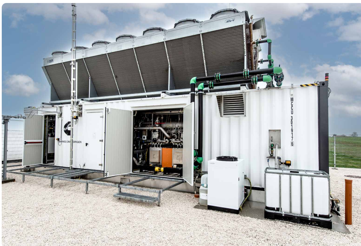
Underground hydrogen storage demonstration facility Rubensdorf, Austria. Photo by kind permission of RAG.
